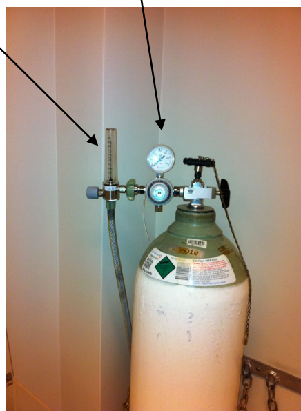
Gas bottle, regulator and flow meter
